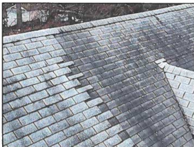
28. Evidence of poor installation
