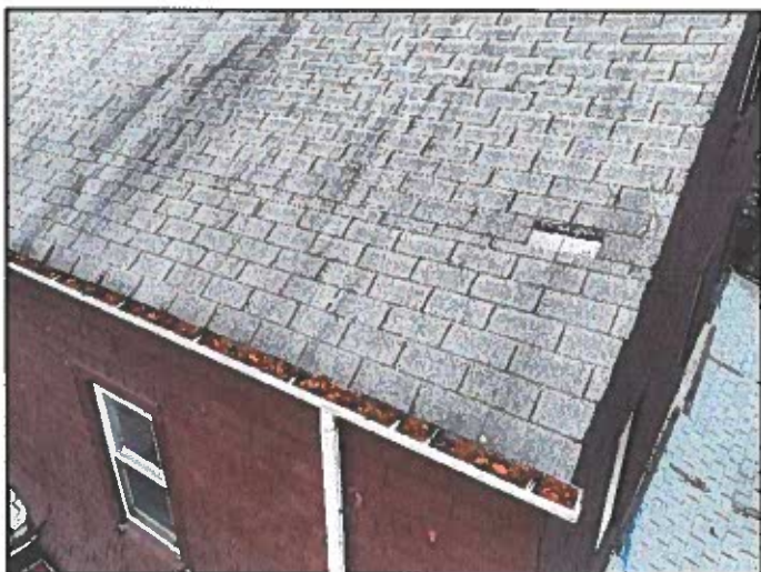
27. Evidence of poor installation
