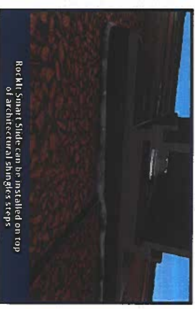
A layer of flexible foam pushes the sealant deep into the shingle granules and around shingle steps
