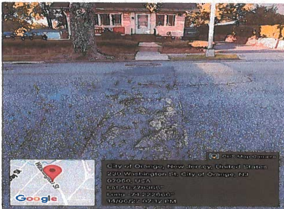
Washington Street (Between N. Essex Ave – E.O. Border) Deteriorated Pavement & Pot Holes
