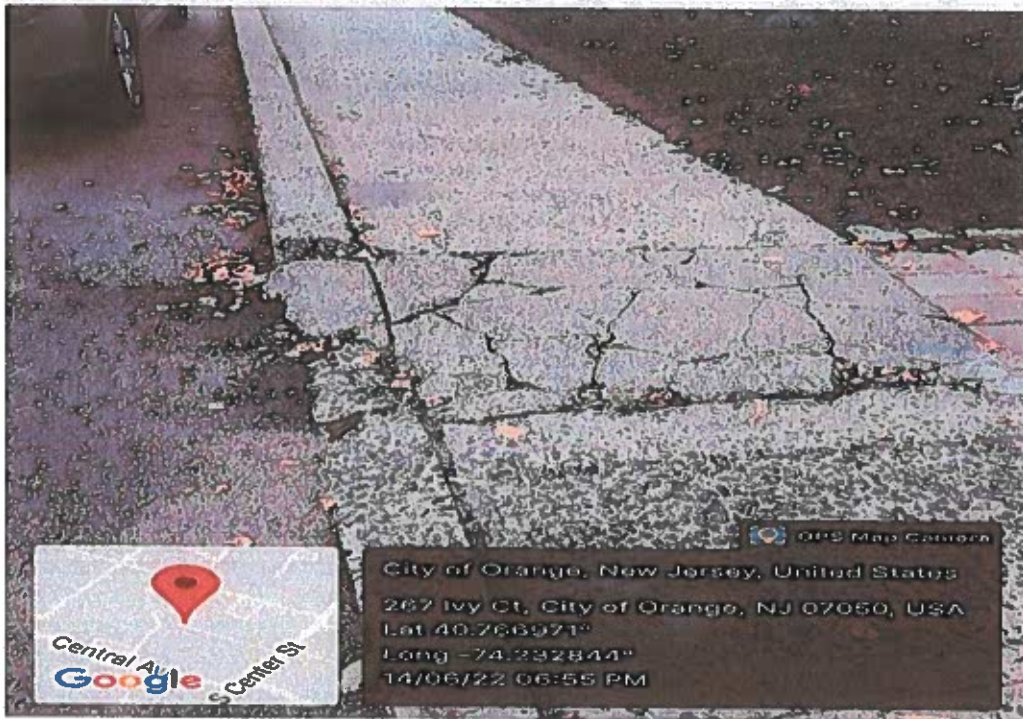
Ivy Court (Between S. Center St – Dead End) Deteriorated Sidewalk & Curb
