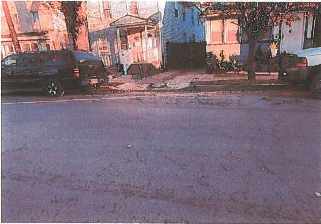
Valley Street (between Union St – Tremont Ave) Deteriorated Pavement, & Sidewalk
