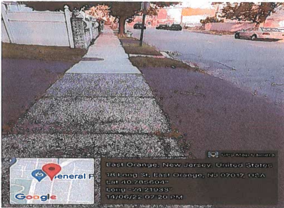
Hayward Street (Between Thomas Blvd – E.O. Border) Cracked Sidewalk
