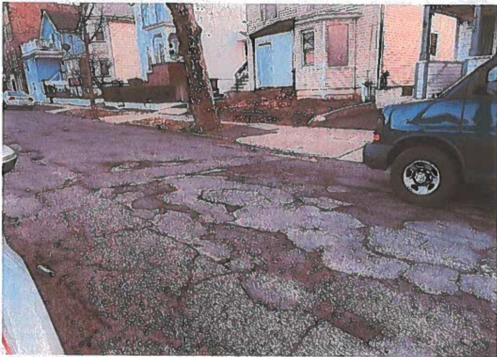
Frankfort Street (between Scotland Rd – Lincoln Ave) Deteriorated Pavement
