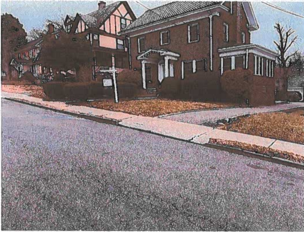
Mountainview Avenue (between Lincoln Ave – Scotland Rd) Deteriorated Sidewalk & Curb
