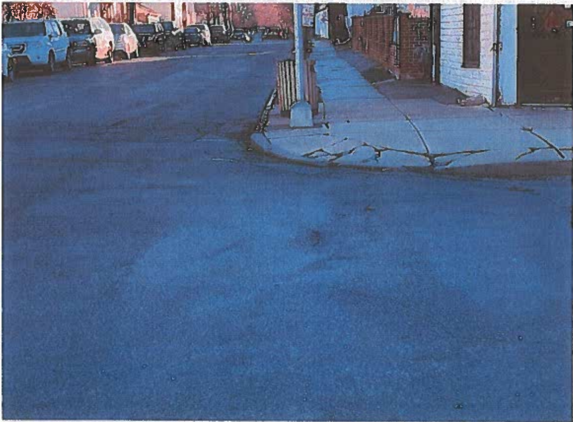
Valley Street (between Union St – Tremont Ave) Cracked Sidewalk & Non-Compliant ADA Ramp
