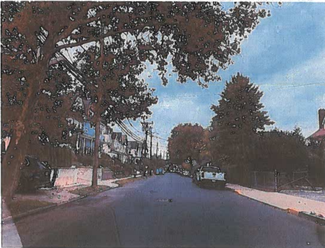
North Jefferson Street (between White St – Main St) Deteriorated Pavement
