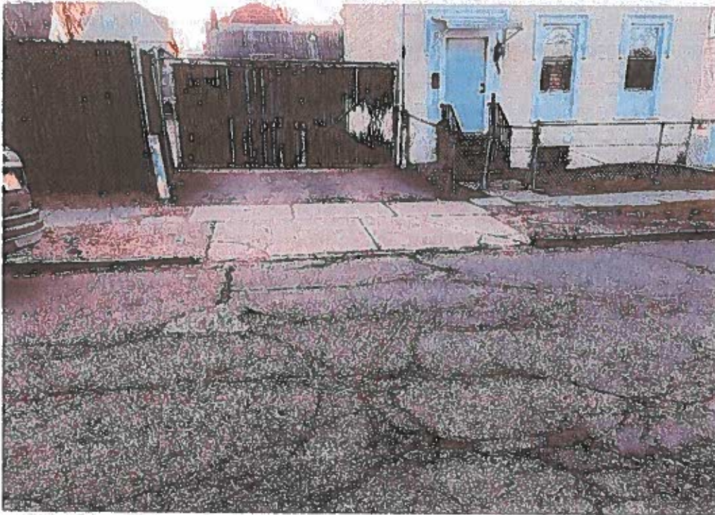
Frankfort Street (between Scotland Rd – Lincoln Ave) Deteriorated Curb & Sidewalk
