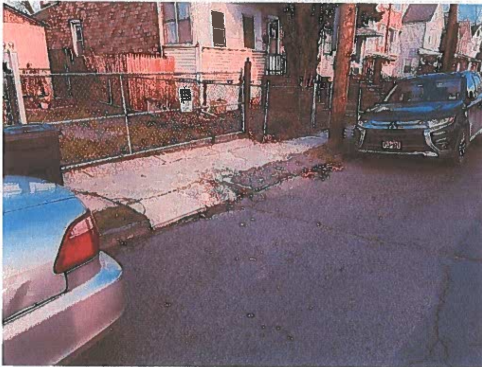
Madison Street (between Bell St – S. Jefferson St) Deteriorated Sidewalk & Curbing
