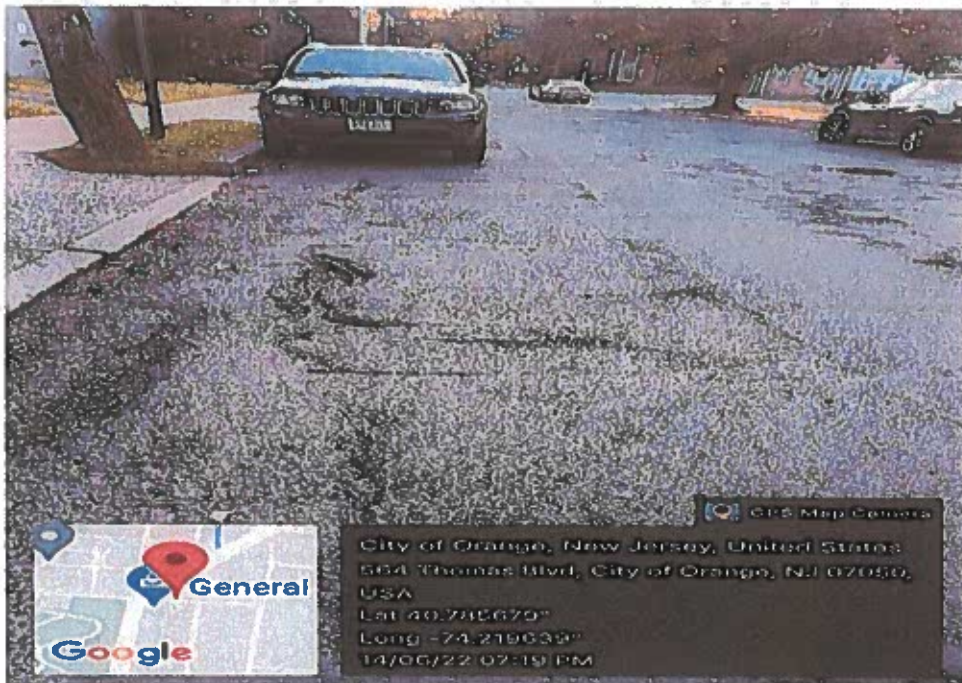
Hayward Street (Between Thomas Blvd – E.O. Border) Deteriorated Pavement
