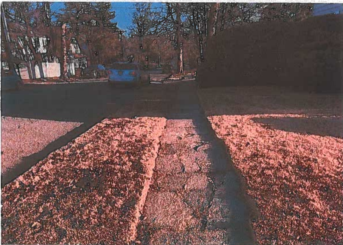
Heywood Avenue (between Berkeley Ave – Mosswood Ave) Deteriorated Sidewalk
