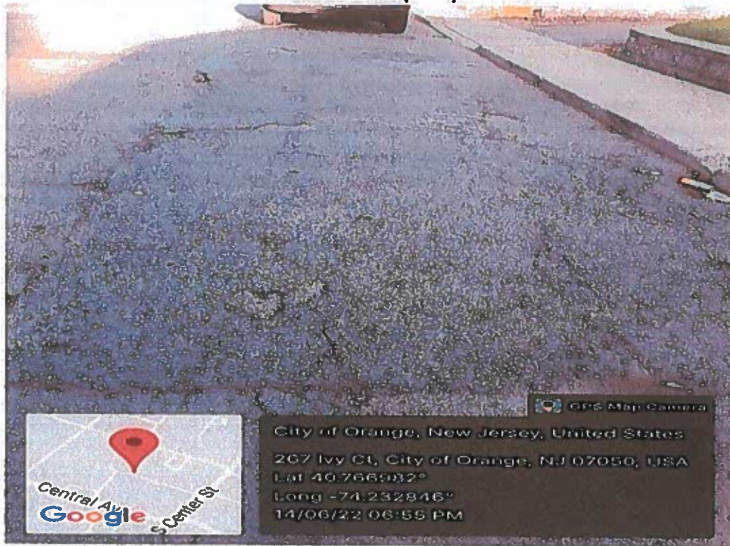
Ivy Court (Between S. Center St – Dead End) Deteriorated Pavement
