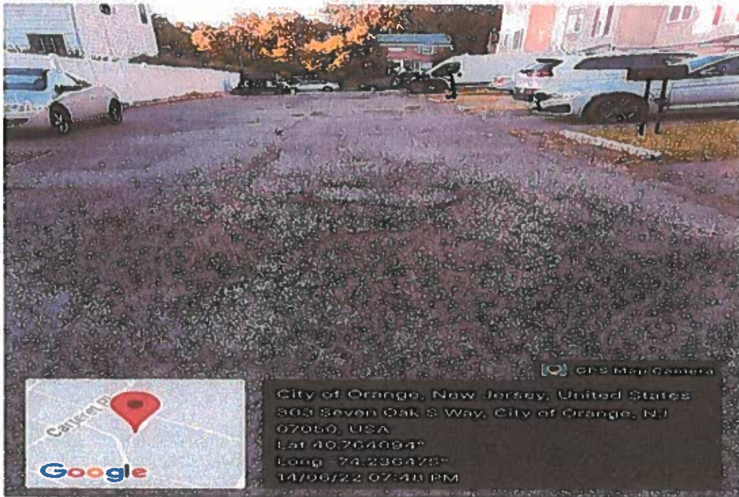
Seven Oaks Way (Between Reynolds St – Dead End) Deteriorated Pavement
