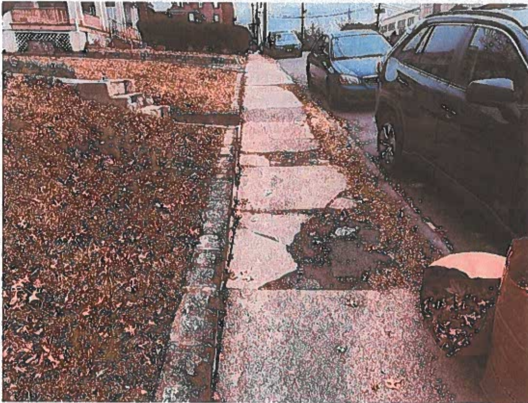
Mountainview Avenue (between Lincoln Ave – Scotland Rd) Deteriorated Sidewalk
