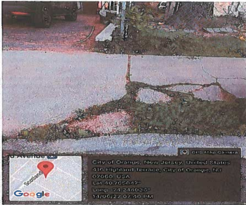
Highland Terrace (Between Highland Ave – Dead End) Deteriorated Sidewalk
