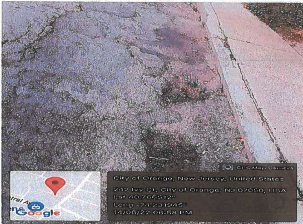
Ivy Court (Between S. Center St – Dead End) Deteriorated Pavement & Pot Holes
