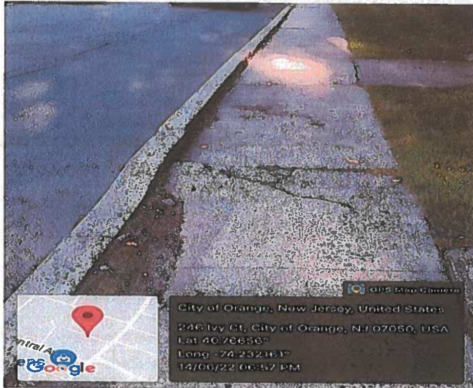
Ivy Court (Between S. Center St – Dead End) Deteriorated sidewalk & Curb
