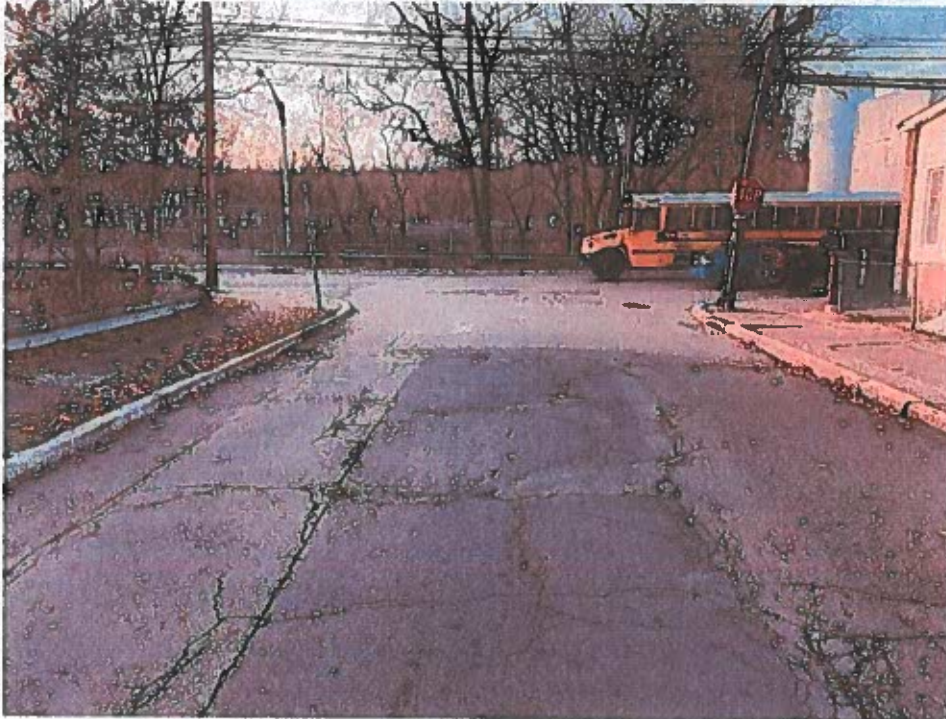
Madison Street (between Bell St – S. Jefferson St) Deteriorated Pavement & Pot Holes
