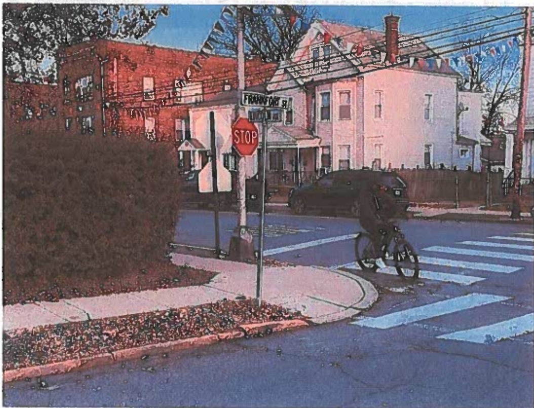
Frankfort Street (between Scotland Rd – Lincoln Ave) Non-Compliant ADA Ramp
