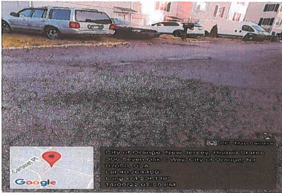
Seven Oaks Way (Between Reynolds St – Dead End) Cracked Pavement
