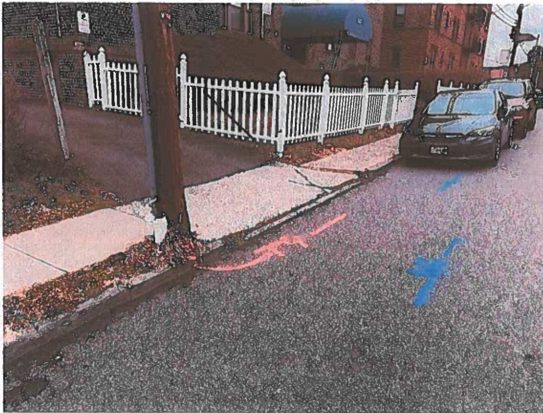
Mountainview Avenue (between Lincoln Ave – Scotland Rd) Cracked Sidewalk Apron & Curb
