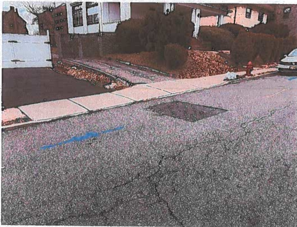
Mountainview Avenue (between Lincoln Ave – Scotland Rd) Cracked Pavement
