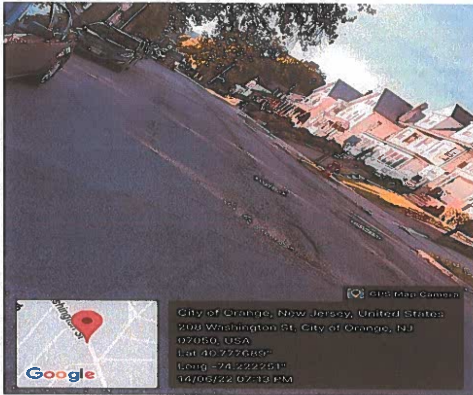
Washington Street (Between N. Essex Ave – E.O. Border) Deteriorated Pavement
