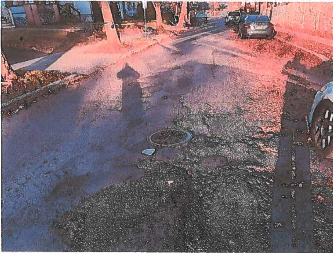
E. Highland Avenue (between S. Center St – E.O. Border) Deteriorated Pavement & Pot Hole
