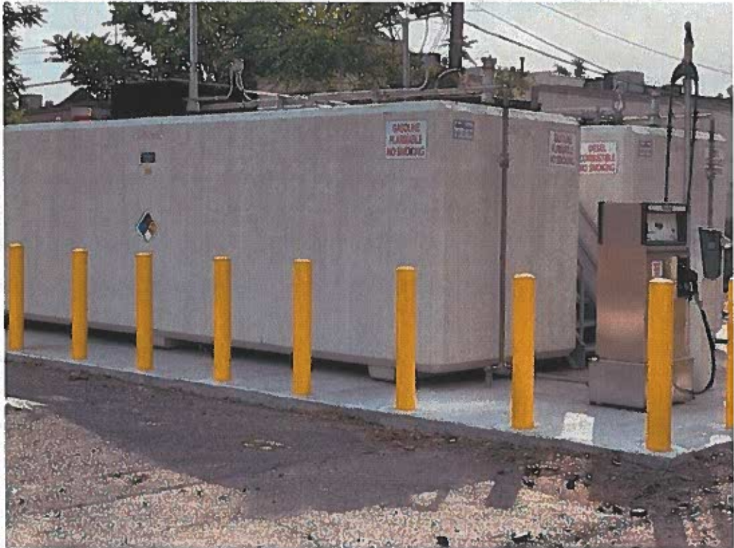
Gas Tanks @ Brook Alley Garage
