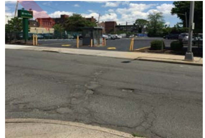
Condition of roadway at intersection of Railroad Place and South Day Street
