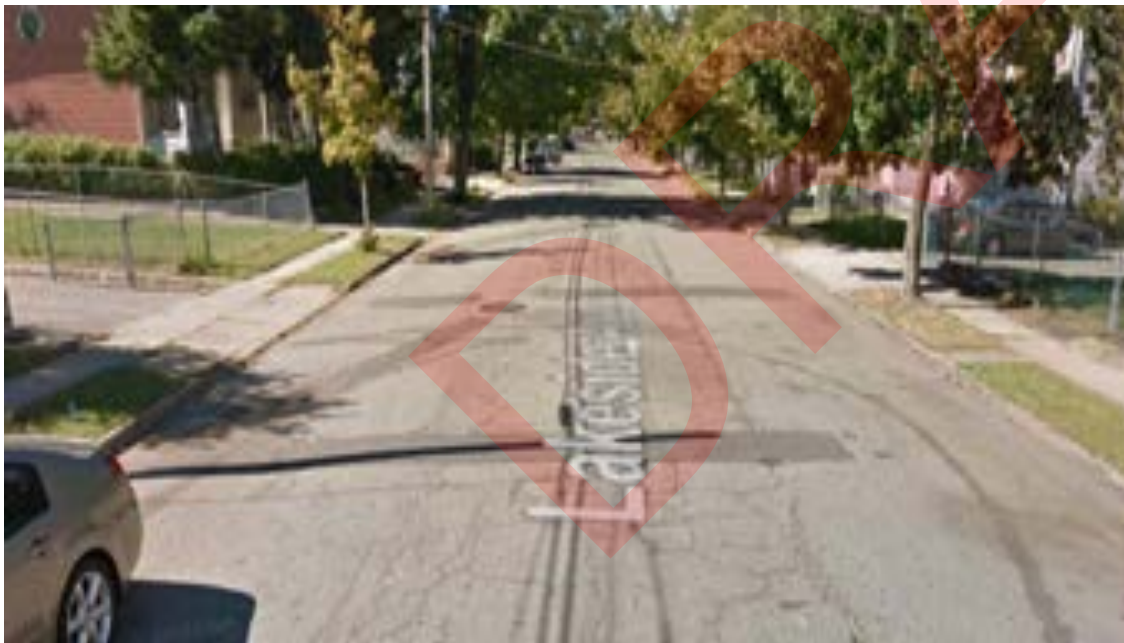
Lakeside Avenue (between High Street and Watchung Avenue) showing extensive alligator cracking and utility trench failure
