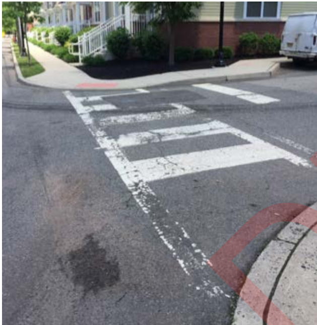
Faded Crosswalk leading to non-compliant ADA curb Ramp
